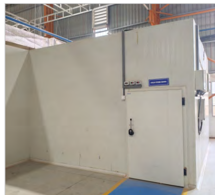
Cold Storage (-18°C)
